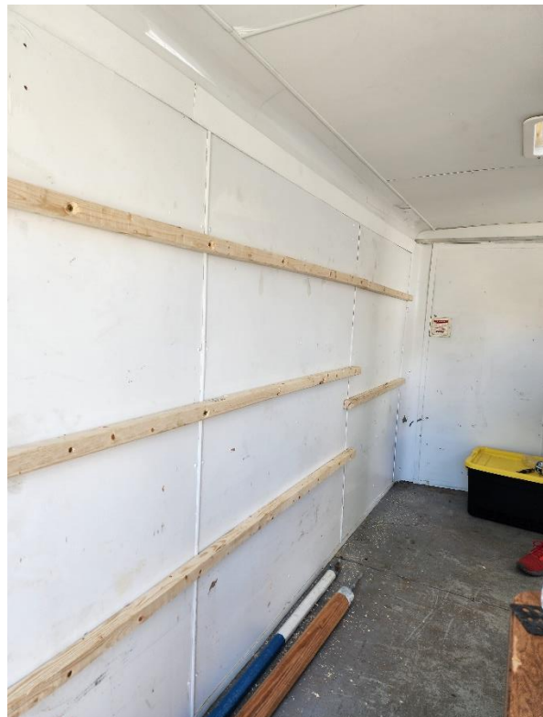
Trailer – View Toward Left Front
