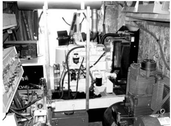
We again had the benefit of central “portable power” from the trailer mounted 50 kW generator provided by Ed Frac, AA9WW.
