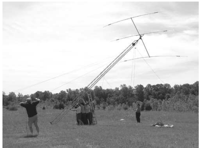
Starting Friday afternoon the radio stations and towers and antenna are put in place. This takes some muscle but is considerably safer and easier with the use of Jim Hillins (KA4UPW) Jeep wench and the tower bases and guys designed and fabricated by Mark Potash (KC9GST).
