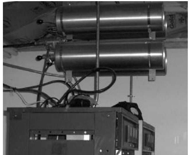
The duplexer (4 pipes in upper part of picture) allows one antenna to receive on one frequency while it transmits simultaneously on a different frequency
