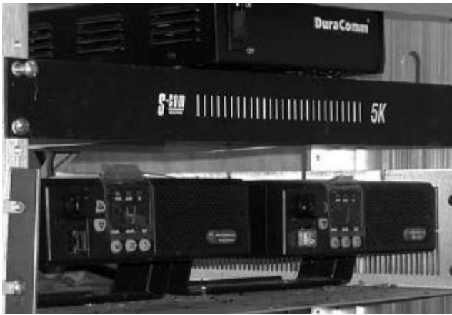
The ORC Link Repeater Receiver (right), Transmitter (left), Controller (middle) and power supply (top)
